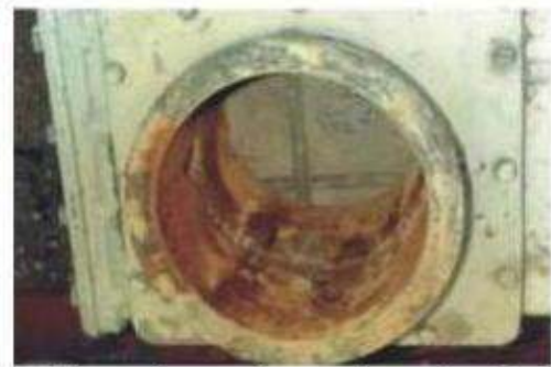
Normal metal seat ring after 2 months in operation
